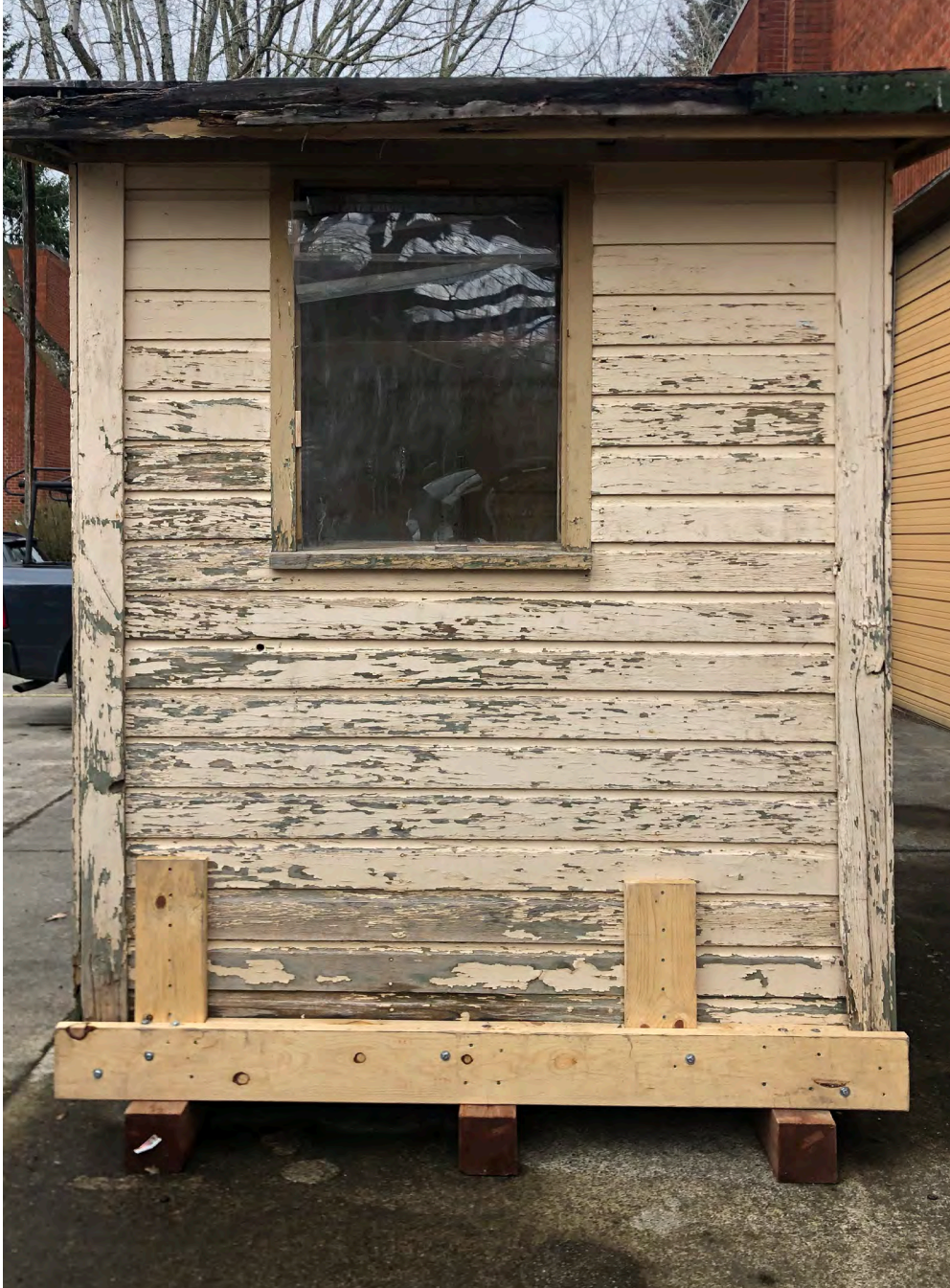
Condition of exterior wall siding and corner trim on the back elevation.
