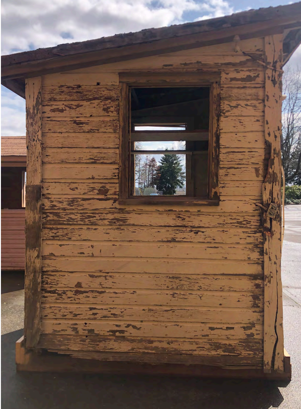
Condition of exterior wall siding and corner trim on the left elevation.
