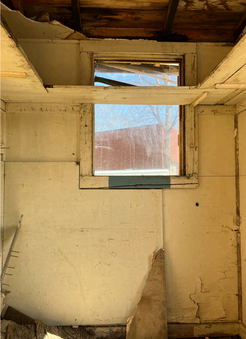
The interior of the back elevation. Note the bare seams between the gypsum board, which is typical throughout the interior of the structure. The gypsum board has moisture-related deterioration in the back right corner and extensive loss of the ceiling boards.
