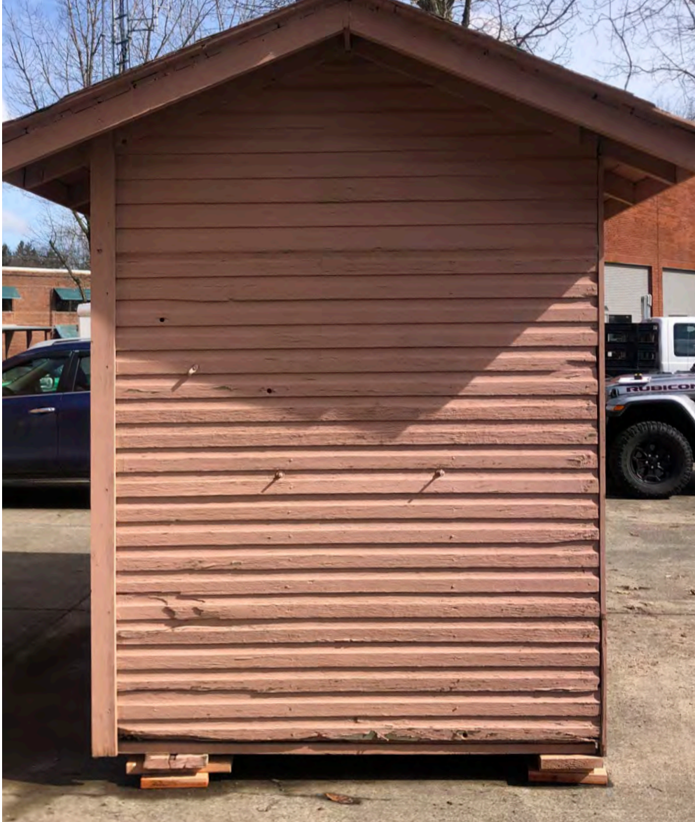
Condition of exterior wall siding and corner trim on the back elevation.
