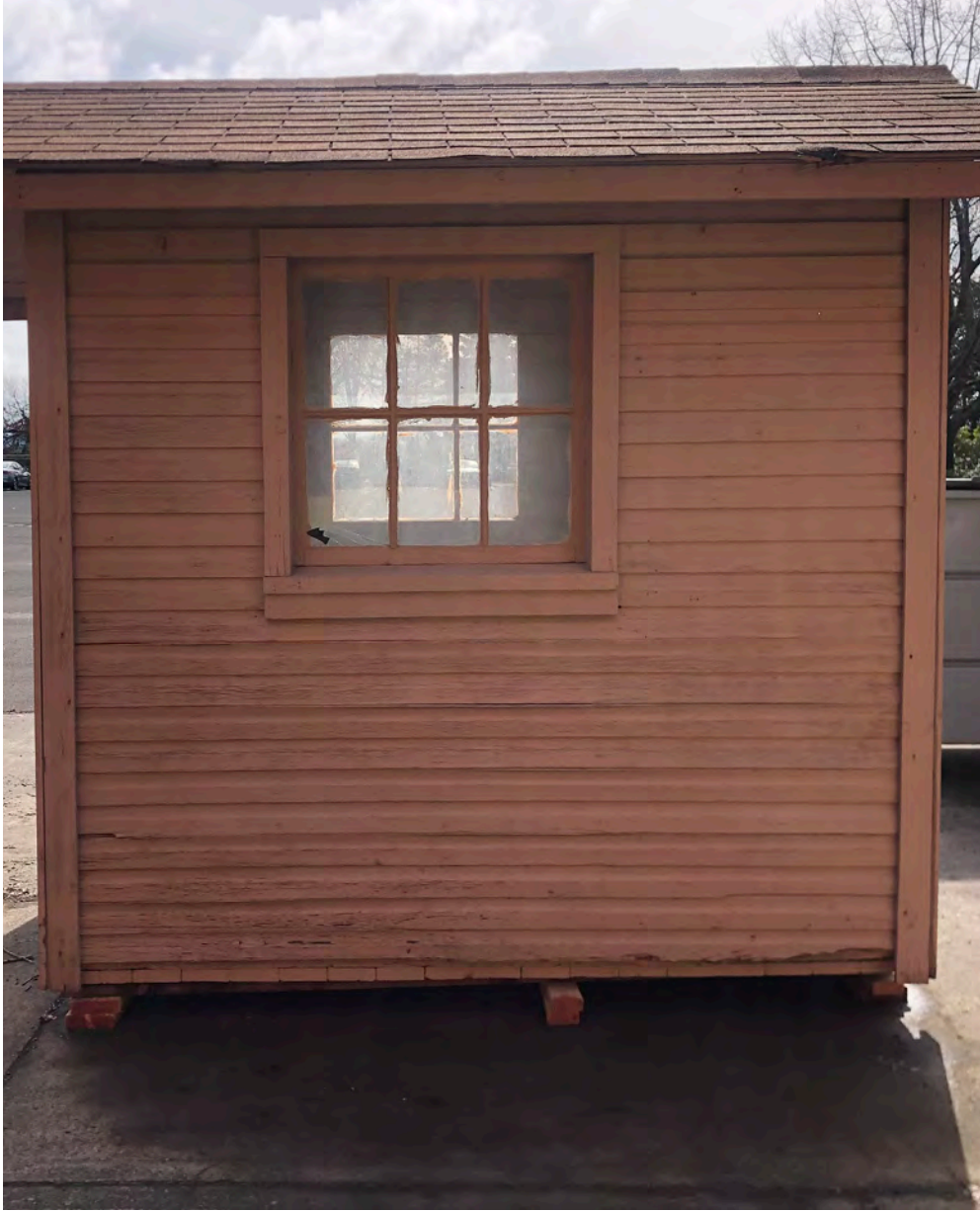
Condition of exterior wall siding and corner trim on the right elevation.
