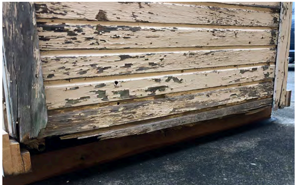
Base of the left elevation, where floor framing damage is damaged and missing toward the back (left) side of the elevation.
