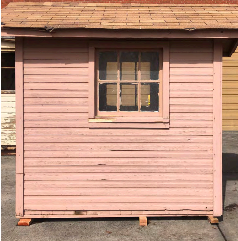
Condition of exterior wall siding and corner trim on the left elevation.
