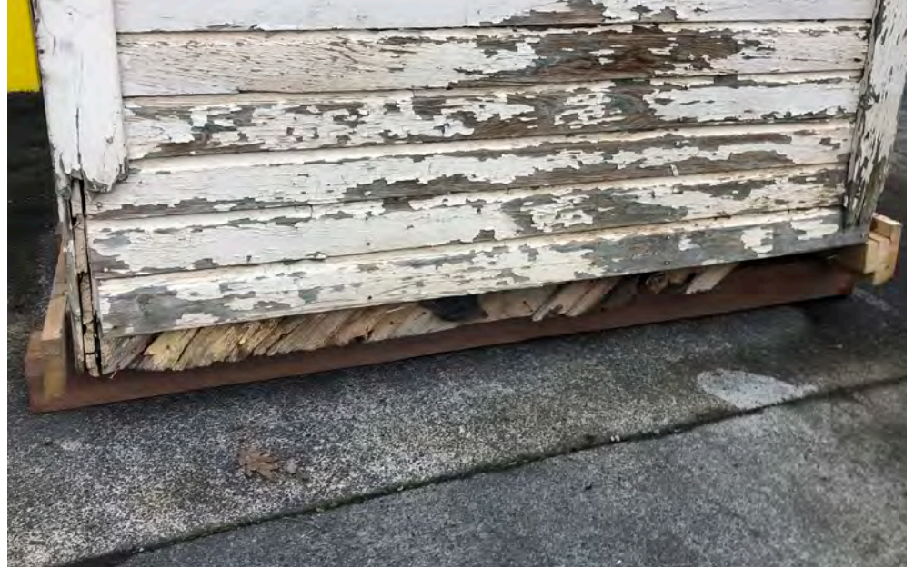
Base of the right elevation, where floor framing damage is damaged and missing toward the back (right) side of the elevation.
