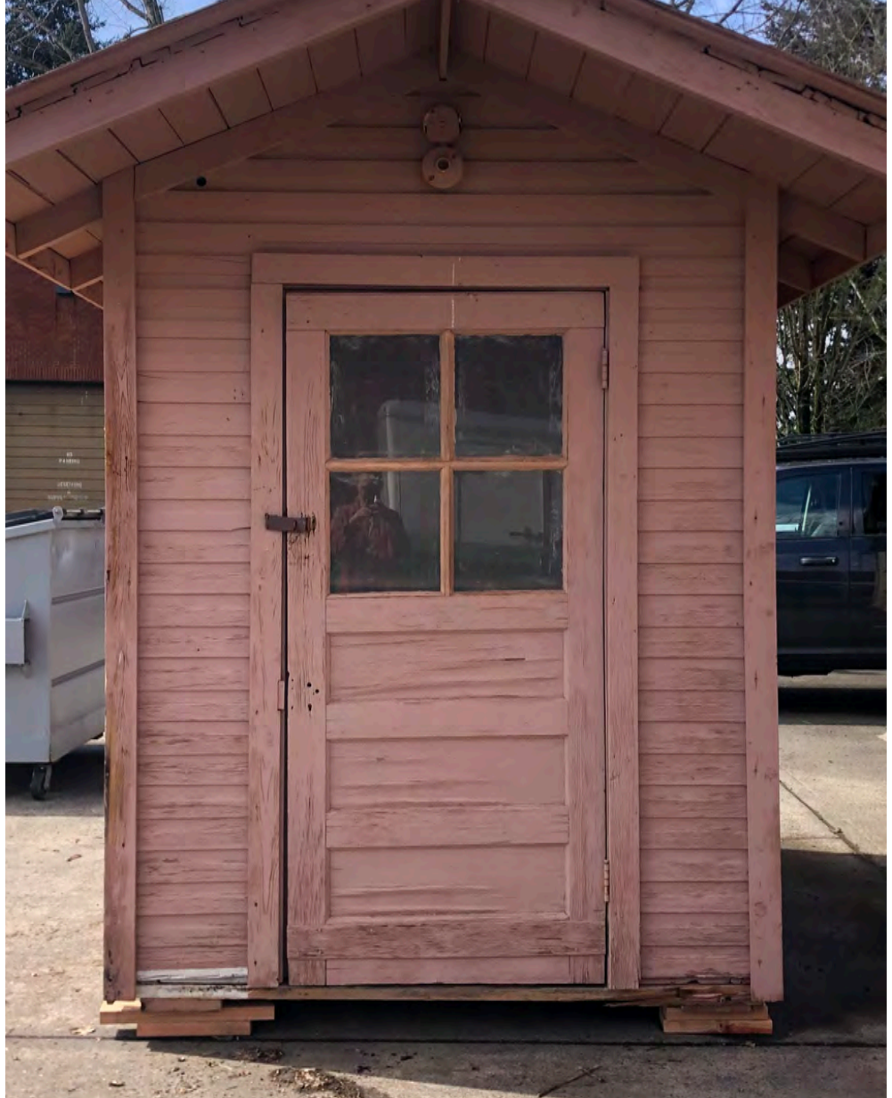
Condition of wall exterior siding and corner trim on the front elevation.
