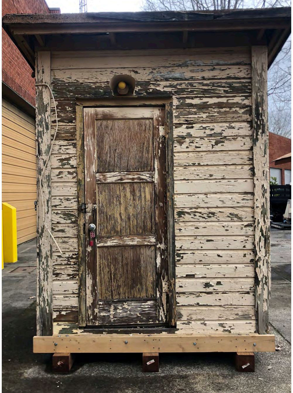
Condition of exterior wall siding and corner trim on the front elevation.
