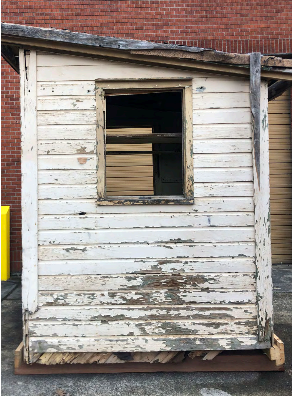
Condition of exterior wall siding and corner trim on the right elevation.
