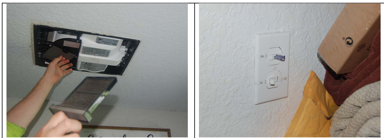
Figure 8. Ceiling-mounted ERV and associated wall switch controls
