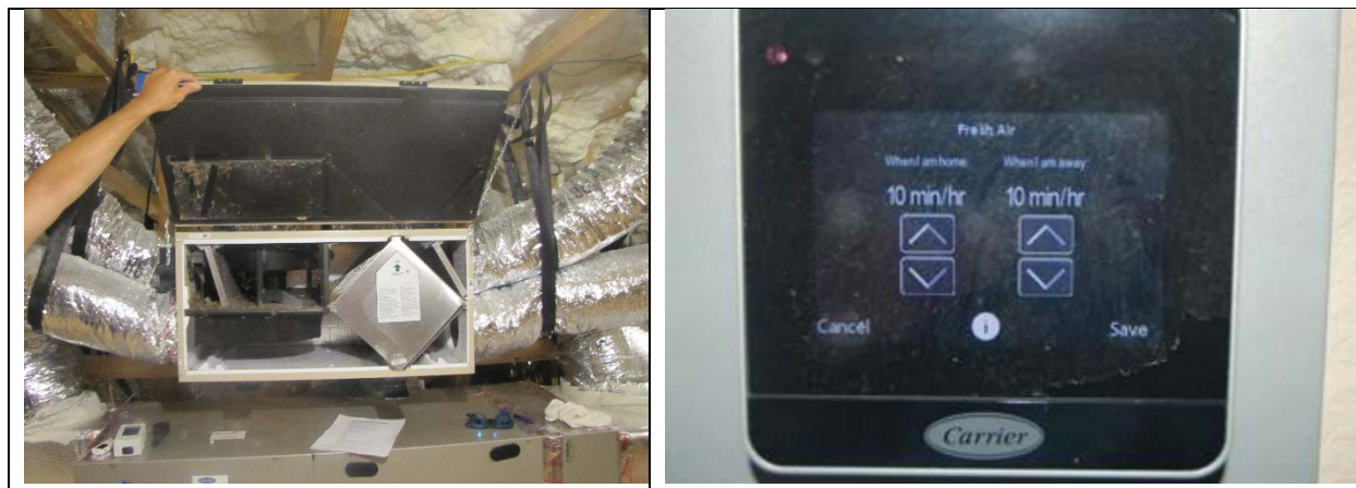
Figure 7. Left – attic-located ERV. Right – associated thermostat control. Dirty filter hindered operation.
