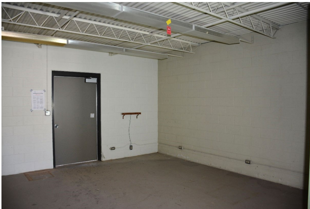
Figure 18. Room 101, showing a grounding busbar near southern entrance (2360_0172, DRI 2023).
