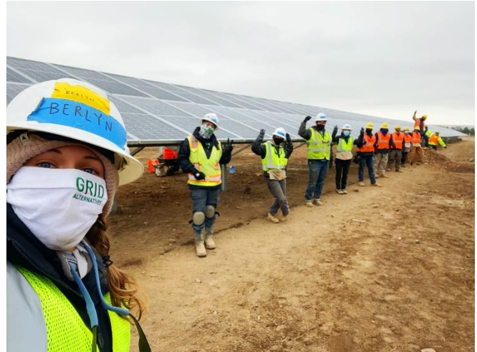
Figure 1. GRID trainees on-site at the Budget Period 1 project site in Boulder, Colorado.
