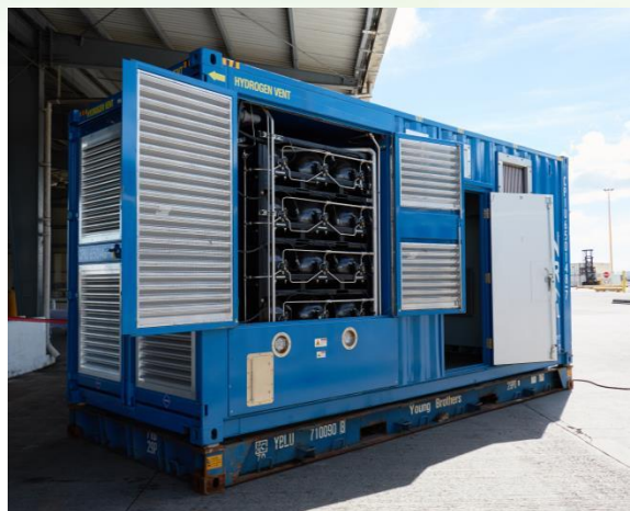
20 foot containerized, 100 kW PEM fuel cell
