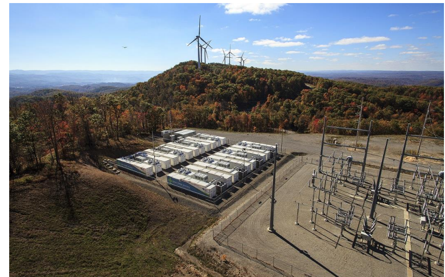
AES 32MW/8MWh grid energy storage solution at the Laurel Mountain facility, Belington, WV Source: https://energystorage.org/
