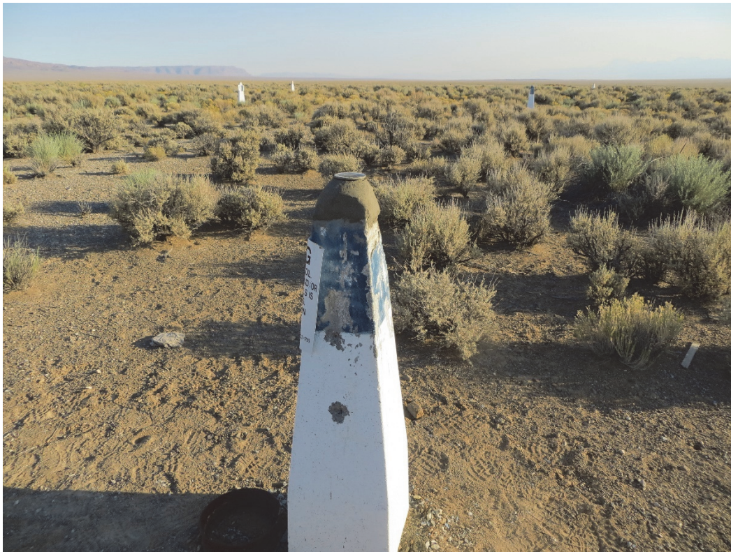
Photograph 7. UC-3 Mud Pit U3E, Showing Repairs Made to the Top of the Monument (view from northeast monument, looking south)
