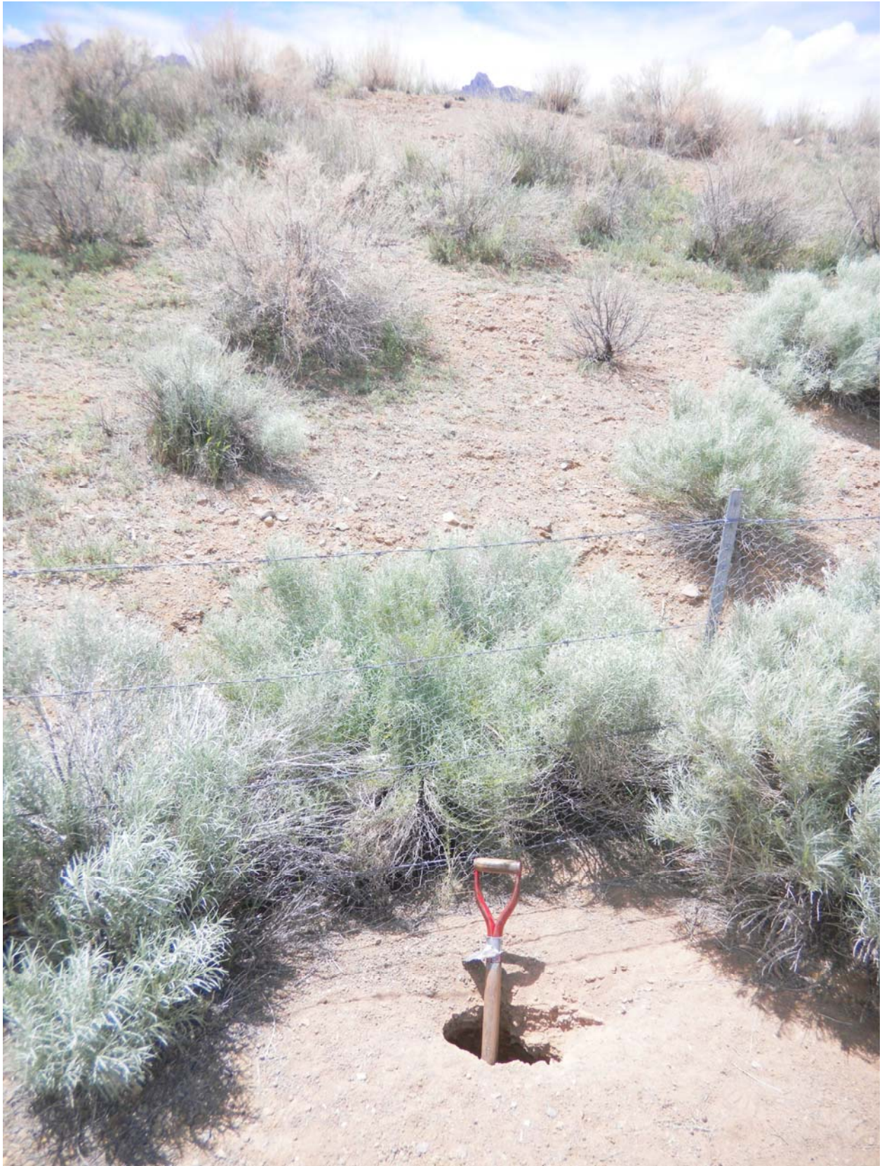
Photograph 13. UC-1, Possible piping structure near east toe of cap
