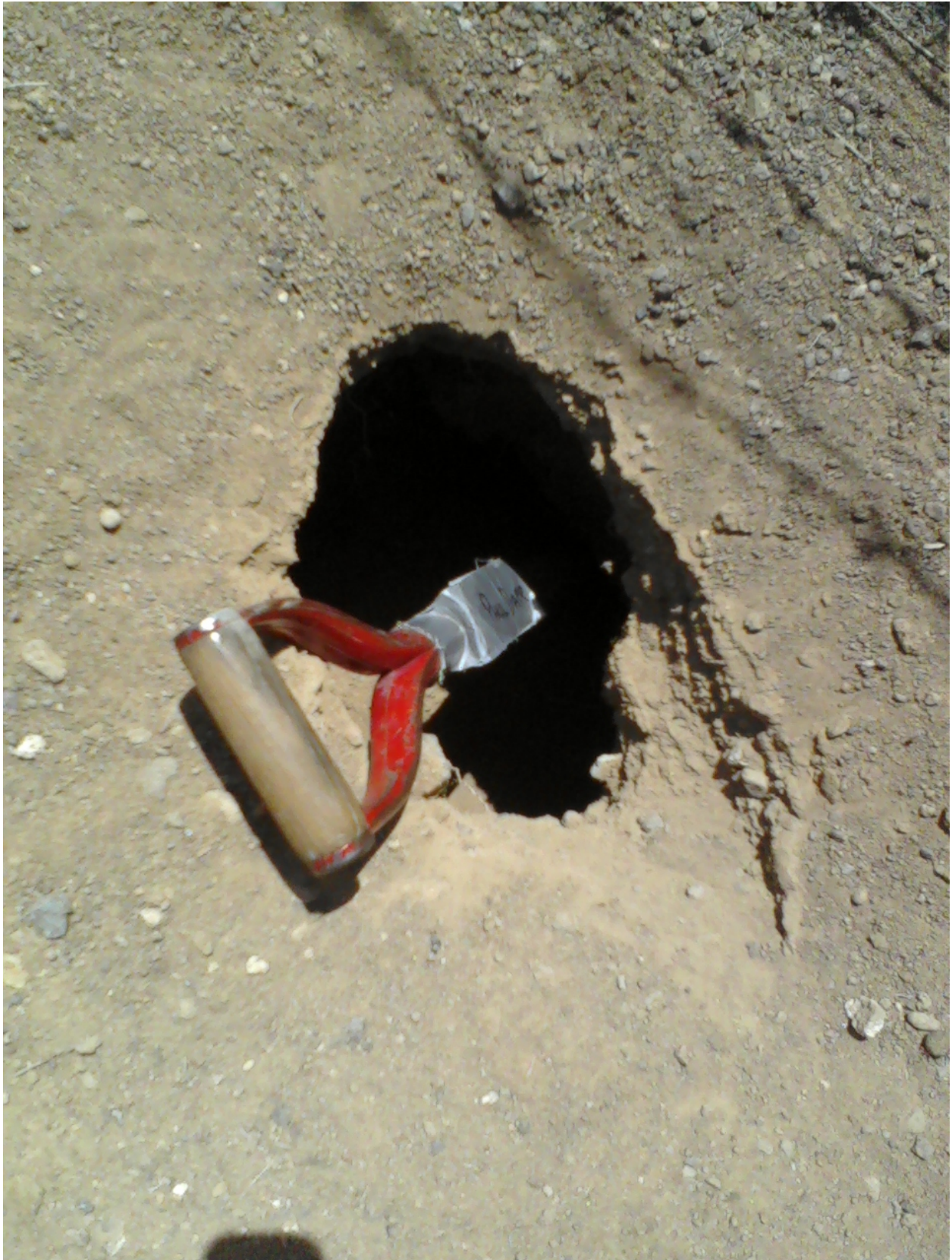
Photograph 14. UC-1, Possible piping structure near east toe of cap
