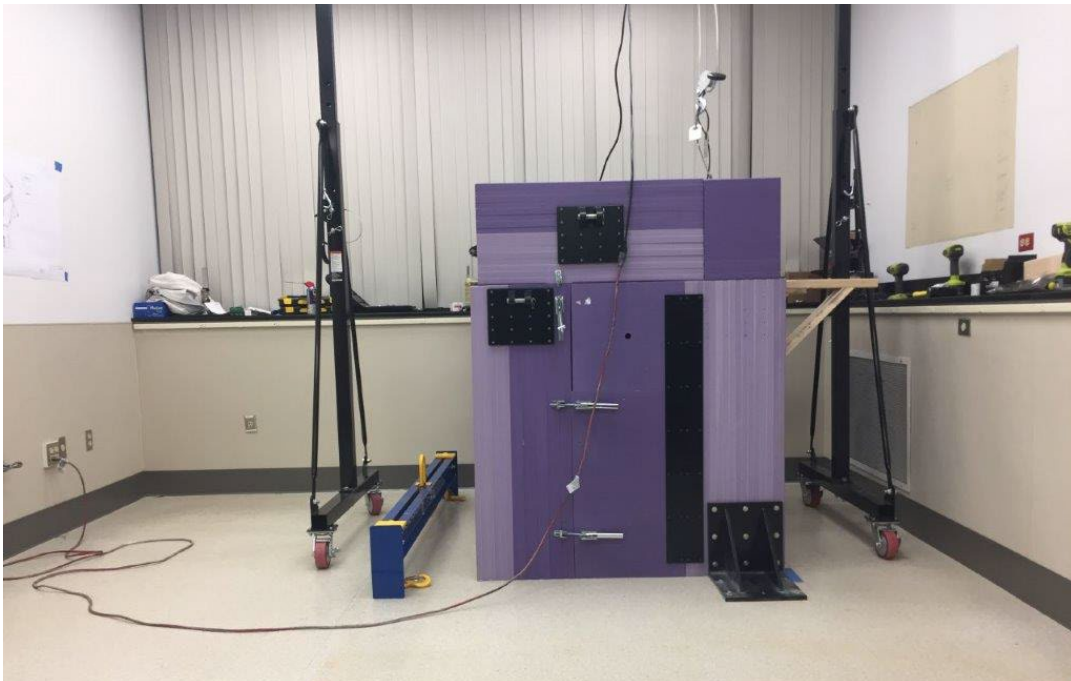
Fig. 14: Installed neutron generator shielding at LSU. Neutron generator will be enclosed within shielding with neutrons emitted through small circular aperture near middle of shielding.
