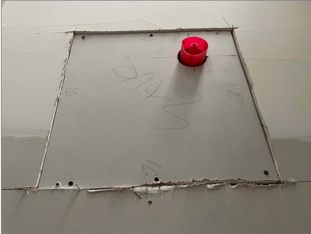
Figure 7. Unsealed ceiling access
