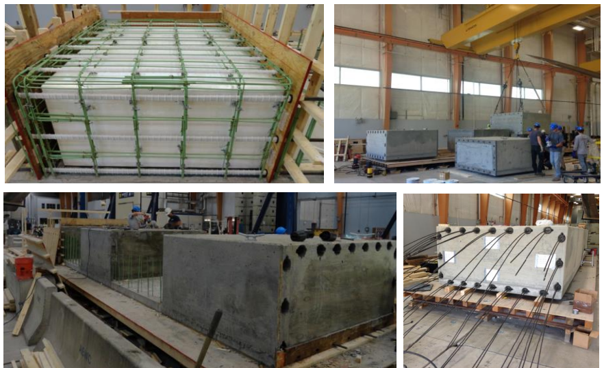
Figure 6 Assembly of 1/4 Scale Prototype of Concrete Hull Member to Demonstrate Modular Construction and to Test Connections
