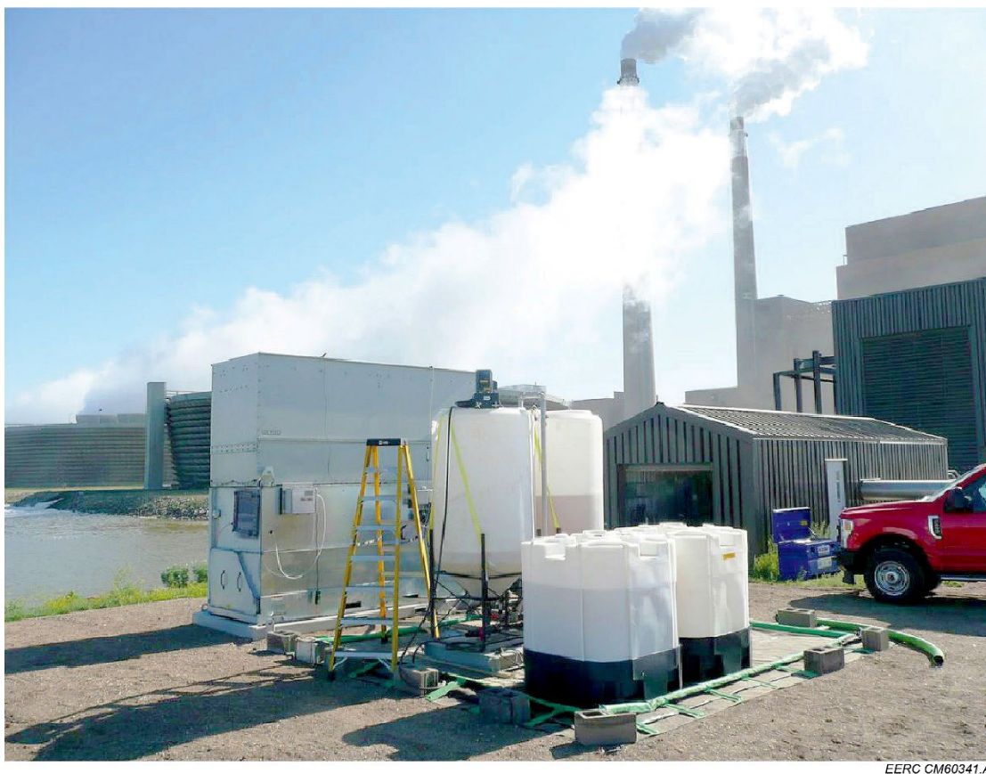
Figure 3. Hygroscopic cooling pilot system during testing at Coal Creek Station.
