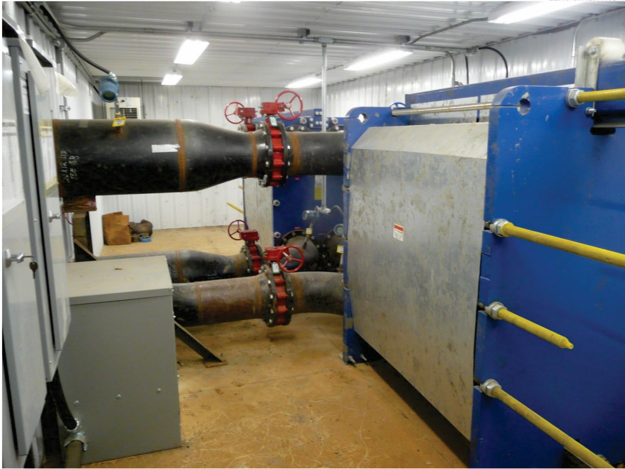
Figure 7. Heat exchanger shed at Coal Creek Station where the plant's condenser cooling water circuit was accessed.
