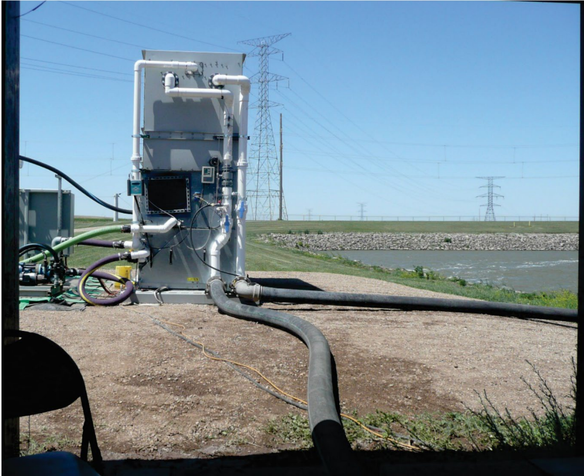
Figure 8. Plant condenser water supply, center, and return pipe to the basin, right.
