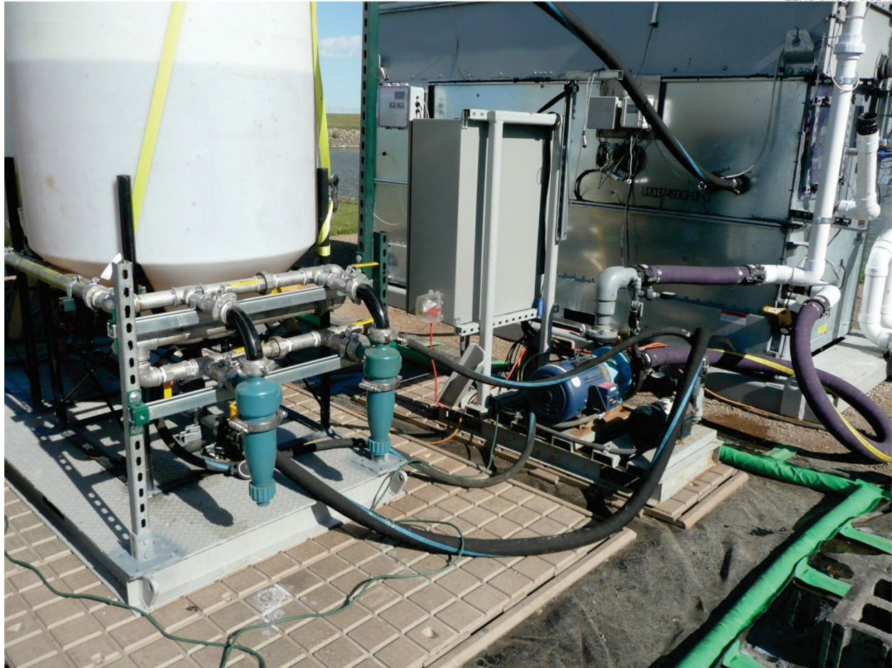
Figure 5. Pump skid, center, and hydrocyclone manifold mounted to the tank skid, left.
