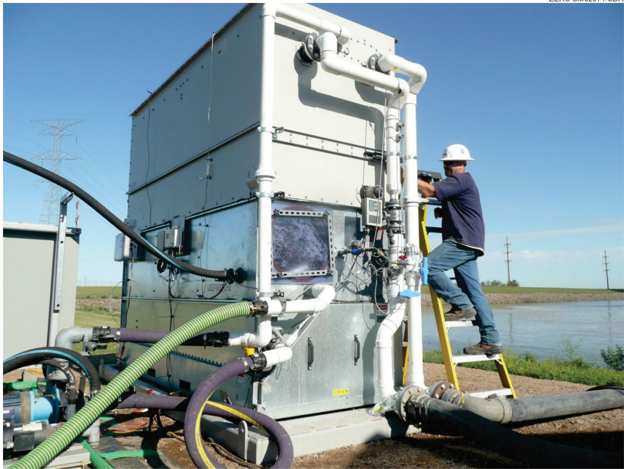
Figure 4. Hygroscopic cooling tower skid during field testing.
