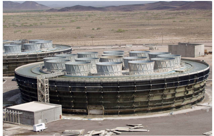
FIGURE 2: Photo of one of the nine Marley Class 700 cooling towers used at the Palo Verde Generating Station.
