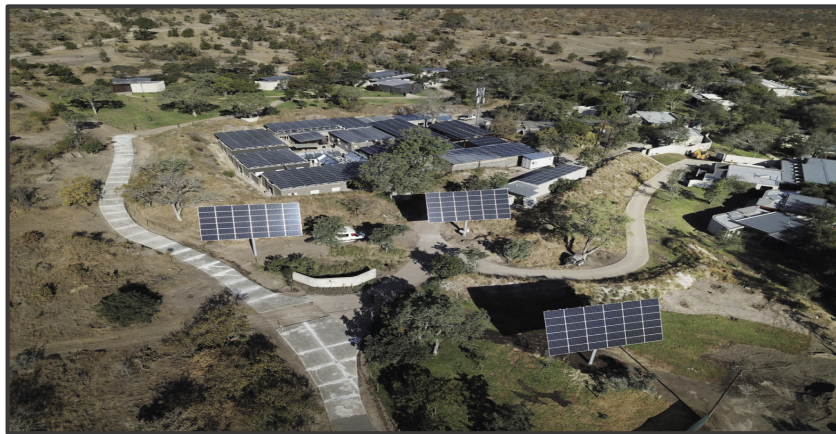
Microgrid in Cheetah Plains Lodge, South Africa's Kruger National Park, featured by 300 kW of PV with 1,027 kWh of Lithium-ion storage capacity and a 150 kVA diesel generator.
