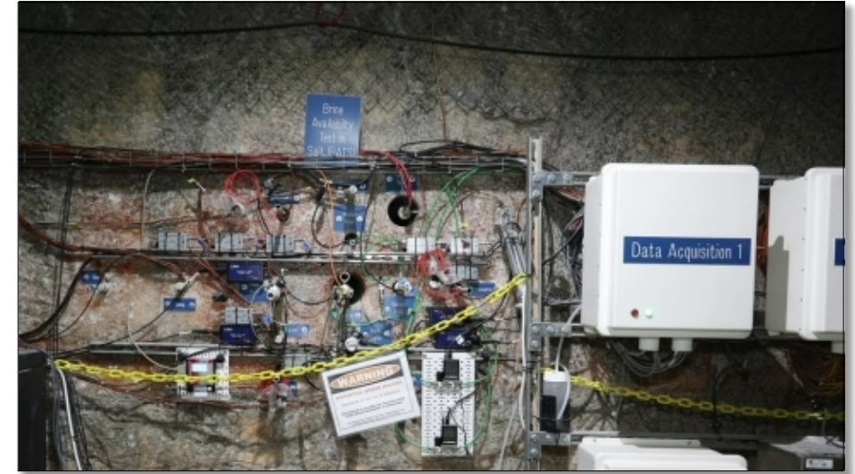
BATS heated array at WIPP
