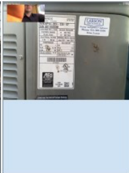
HVAC Unit 2 plate
