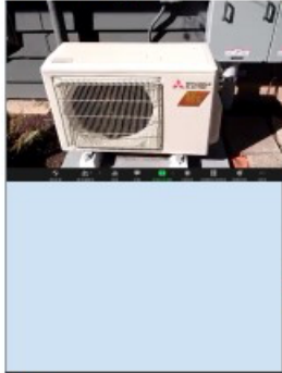
HVAC Unit 3 photo
