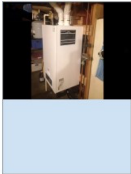
HVAC Unit 4 photo
