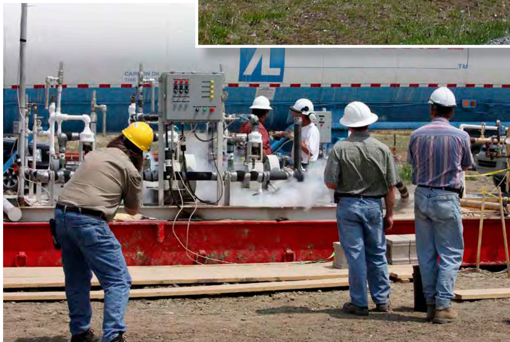
CO 2 injection skid and storage tank at the Tanquary coal test site.
