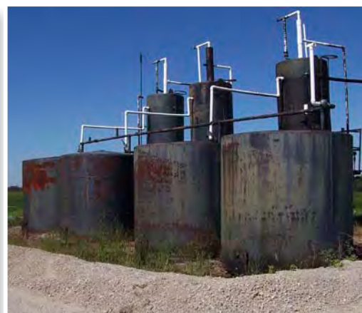
Oil tank battery.
