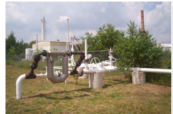
CO 2 pipeline from a gas processing plant in Michigan.
