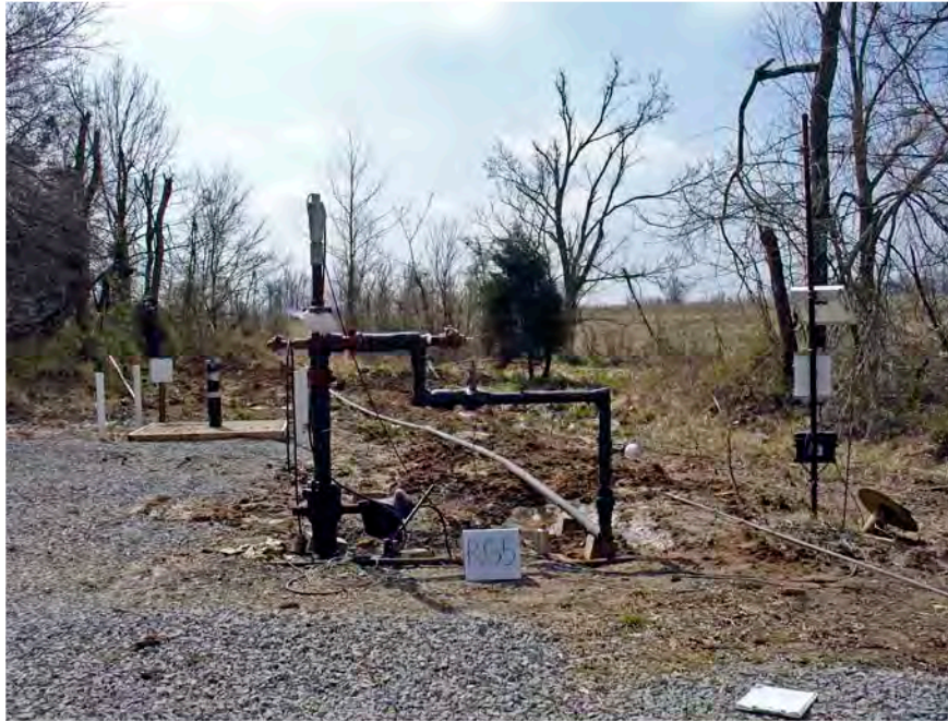
CO 2 injection well at the Sugar Creek EOR III site.
