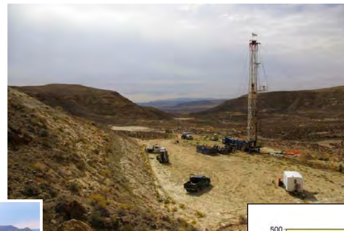
Installation of subsurface geophone array at the Aneth Oil Field, Utah.
