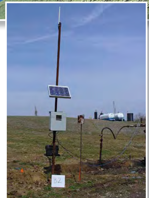
Solar-powered data collection system, Mumford Hills EOR II site.
