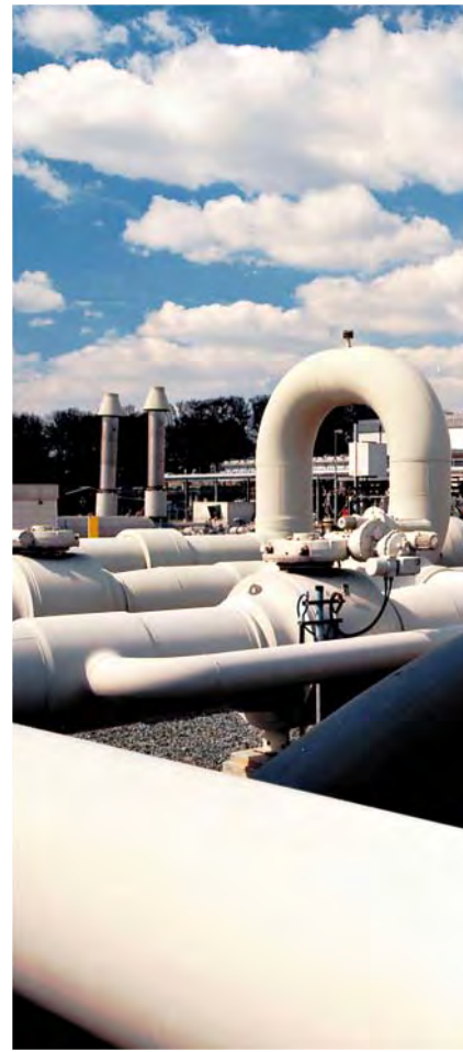
Gas plant infrastructure.
