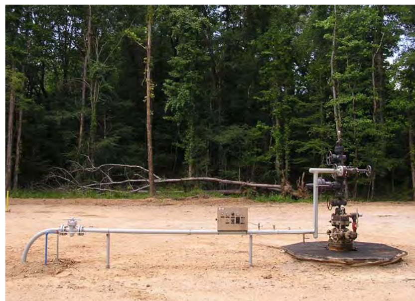
CO 2 -EOR production wellhead. (Courtesy of BEG, UT Austin)
