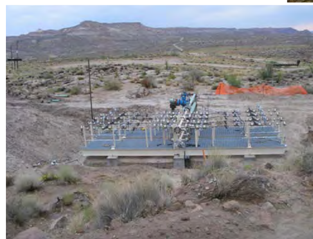
Injection headers at the Aneth Oil Field, Utah. Each valve controls the injection of CO 2 to an individual well.
