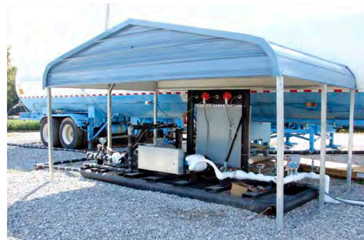
Injection pump skid with CO 2 supply tanker in the background, Mumford Hills EOR II site.
