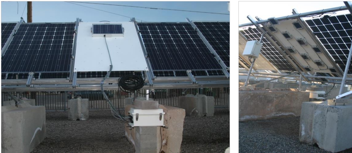
Figure 21: (left) Front side of the IDM placed in the middle of a row of modules. (right) Back side of the IDM.
