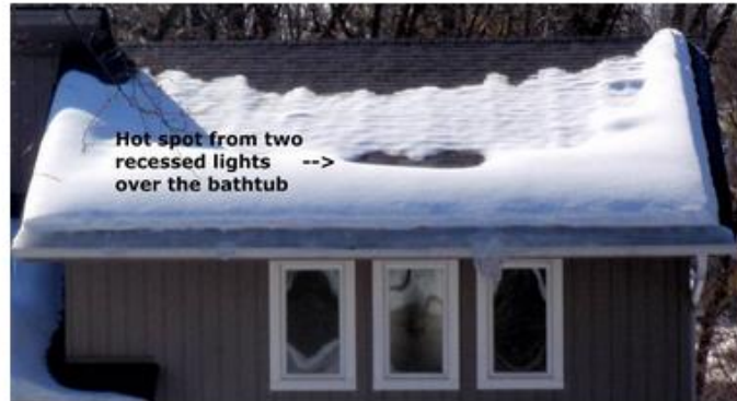
Fig. 5 Excessive Humidity Damages Attic (Source: http://www.hankeyandbrown.com/icedams )
