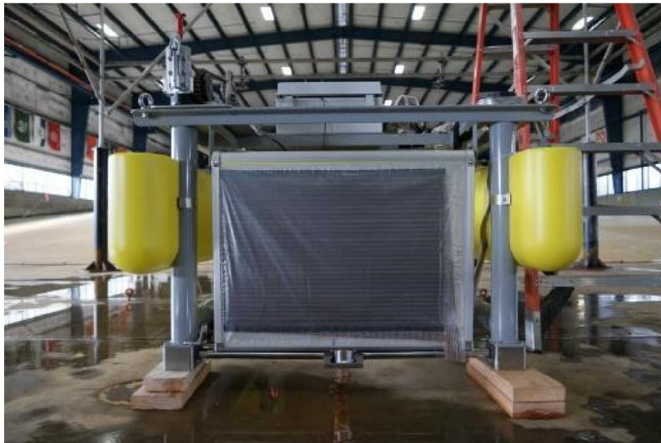
Figure 3-10. Installed Pressure Mat (Phase 1)
