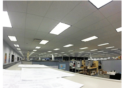
U.S. Toy retrofitted 470 troffers at its corporate headquarters, as part of a lighting upgrade that cut energy use by 54,000 kWh and improved employee satisfaction with work space lighting. Photo courtesy of U.S. Toy Company.
