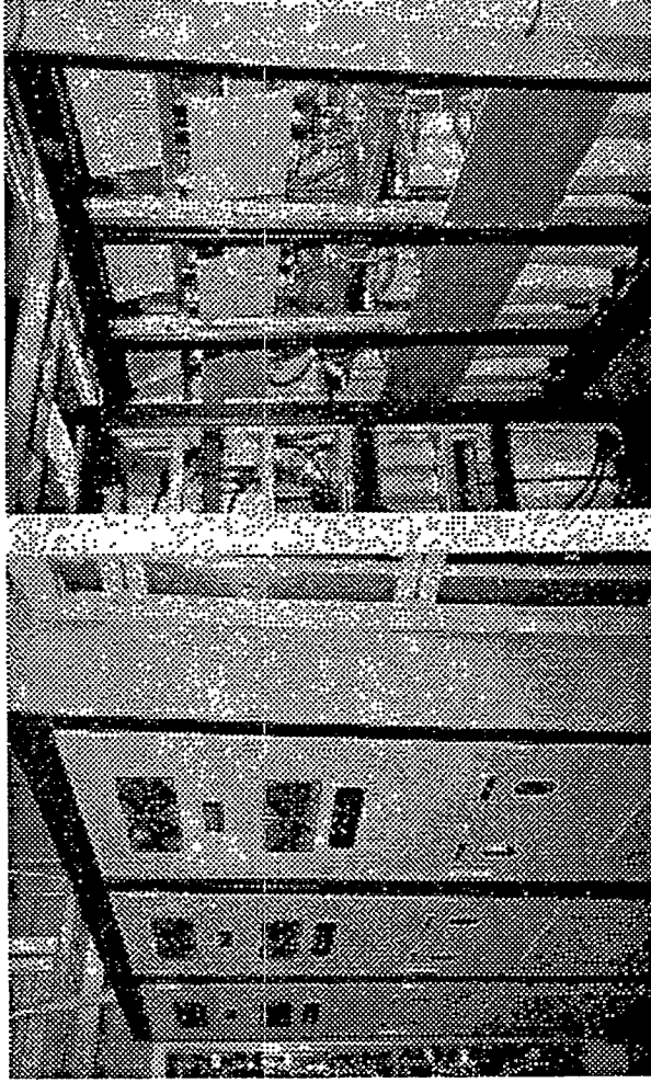
Three 50kW cabinets Center Assembly
