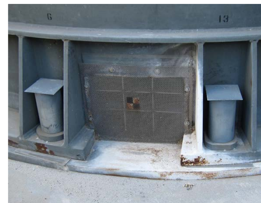
Salt deposition and corrosion at sea-side inlet vents (Diablo Canyon)
