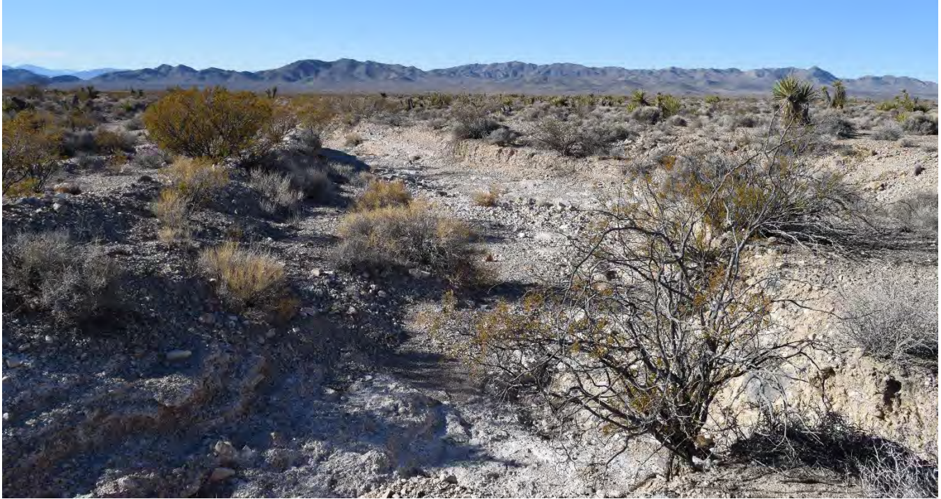
View of a drainage trench that has widened over time along a curve near the sewage lagoons and Jackass Flats Highway.
