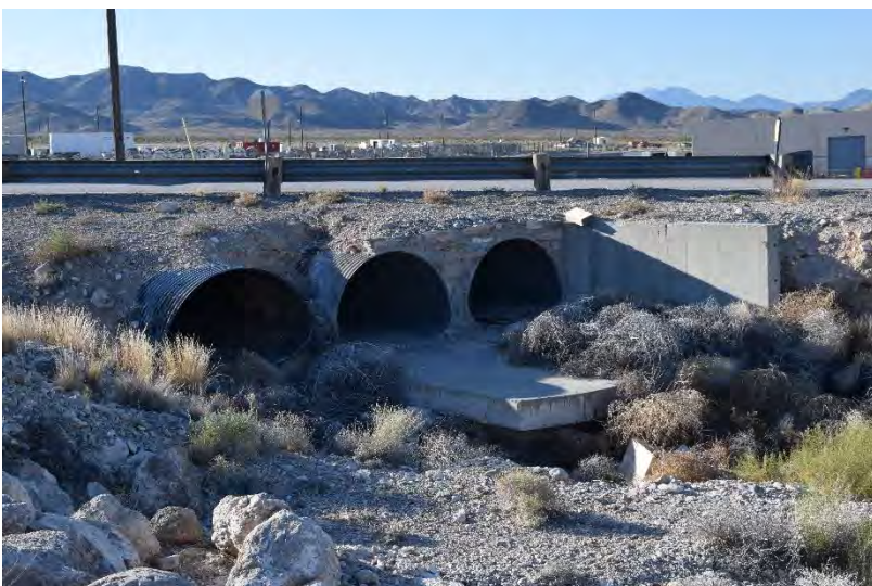
Outflow of Culvert NO1 with masonry retaining wall. Direction facing: East-southeast Photographer: King Date: 2017
