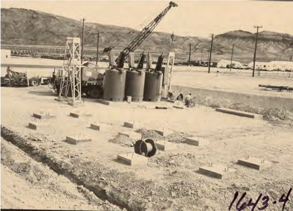
The foundations seen in this photo are still present as of 2017. (See current photo below, taken from a similar angle.) Elevation: N/A Direction facing: North-northwest Photographer: REECO 1982 (Photo # 1643-4) Date: 1963
