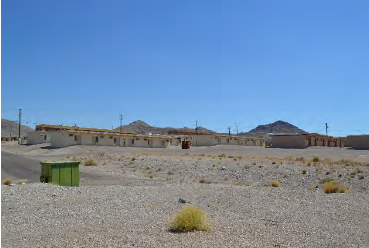
Culvert JA1 is under driveway visible above trash container. Direction facing: Northeast Photographer: Menocal Date: 2017
