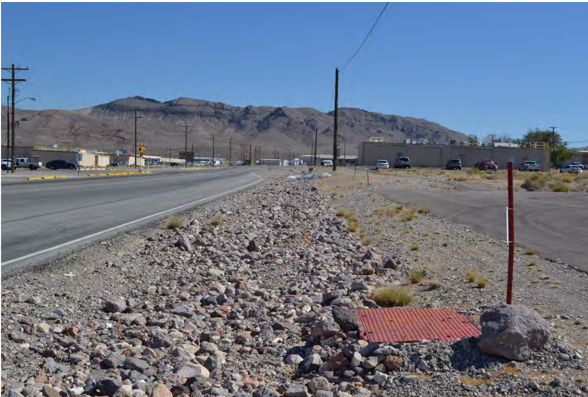
Drainage with riprap on east side Mercury Hwy. Direction facing: North Photographer: Menocal
