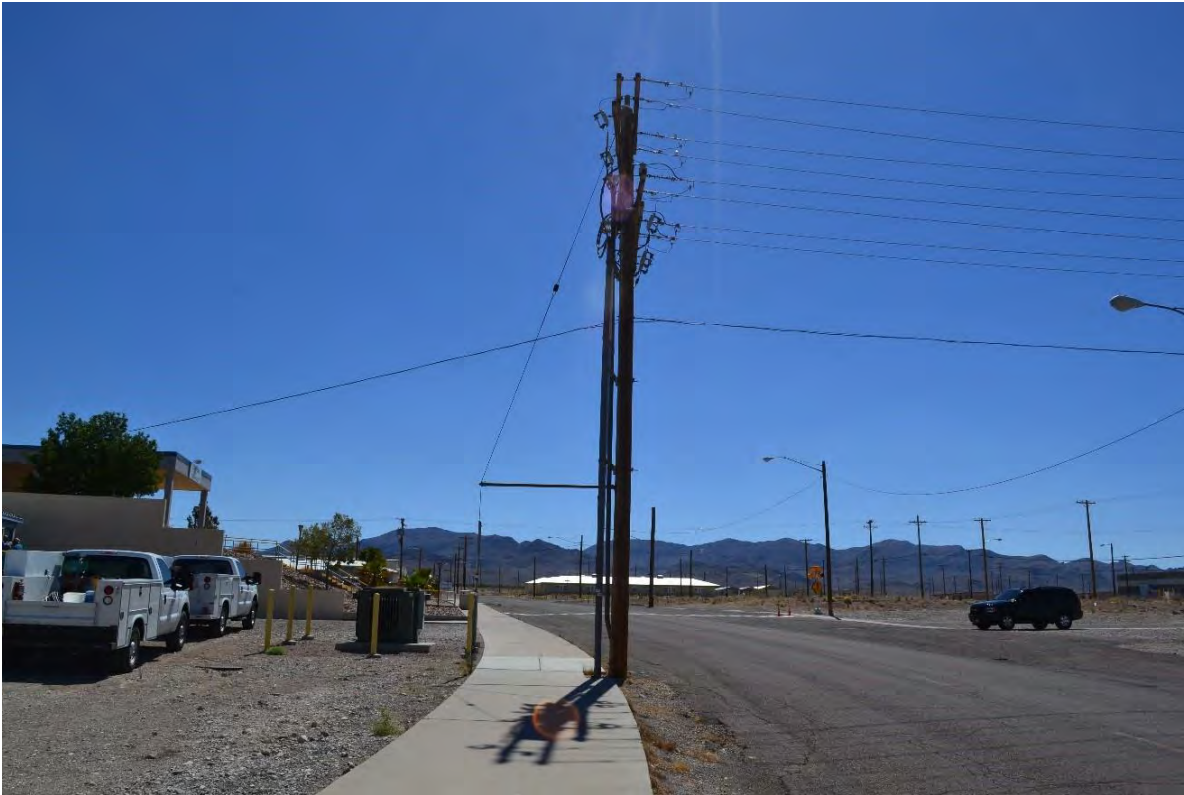
One of the few curbs found in Mercury, located on the north side of Ranger Ave. in front of the cafeteria. Direction facing: East Photographer: Menocal Date: 5/24/2017
