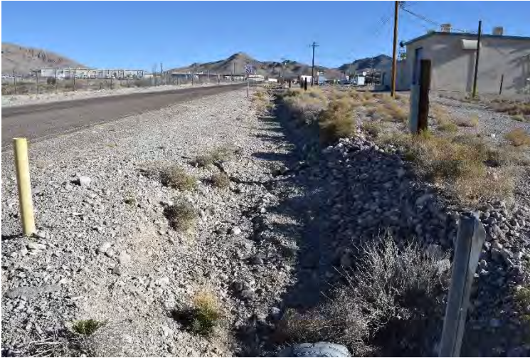
View from Culvert SJ2 toward SJ1. Direction facing: Northeast Photographer: Menocal Date: 2018
