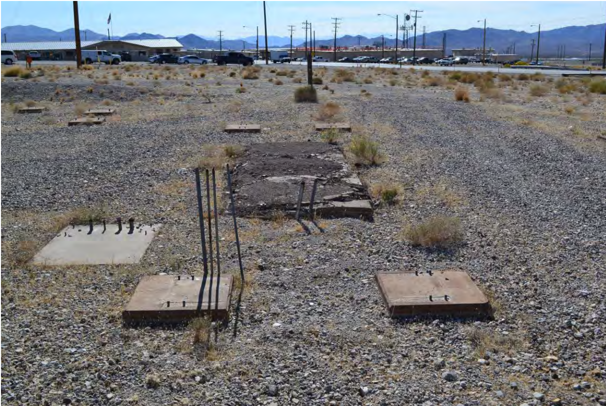
Elevation: N/A Direction facing: Southwest Photographer: Menocal Date: 10/17/2017
