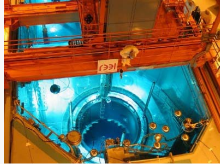
Open PWR Pressure Vessel for Fuel Handling Operations
