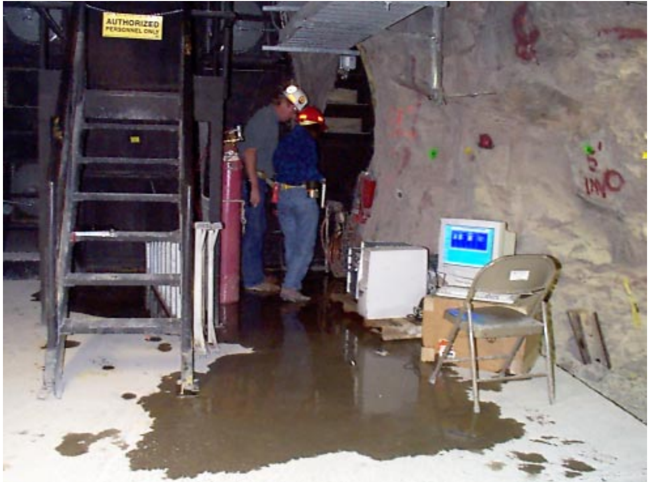
Figure 21. Condensation observed on bulkhead; puddle on floor in front of bulkhead.
