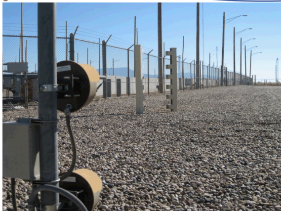
Perimeter Intrusion Detection & Assessment System (PIDAS)
