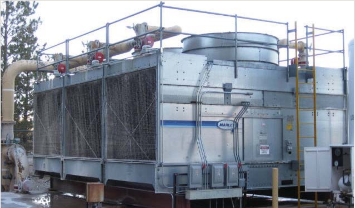
The cooling tower is the core of the system.
