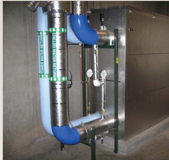
The cold plate heat exchanger uses the cold tower water that is produced in the winter to cool the chilled water in the building.
