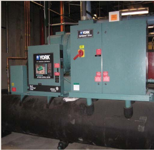
During the winter, when the outside temperature is low enough that the cooling tower can produce 45°F water, the chiller remains off. This reduces the electrical consumption for process and computer rooms by as much as 50%.
