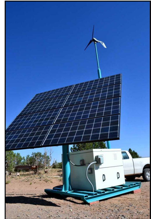
1080 W PV-wind hybrid system on residential unit in Kayenta, AZ
