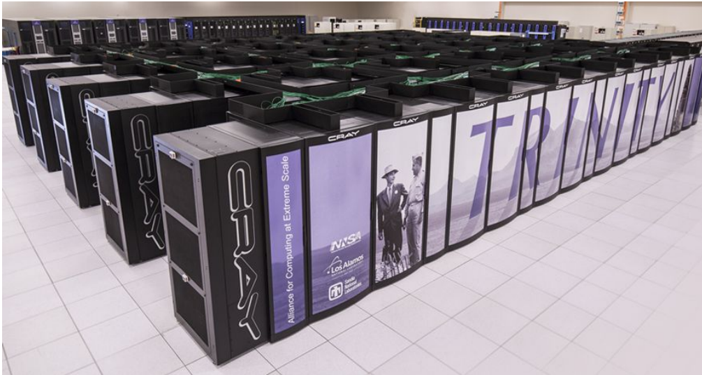
Trinity Supercomputer at Los Alamos National Laboratory
