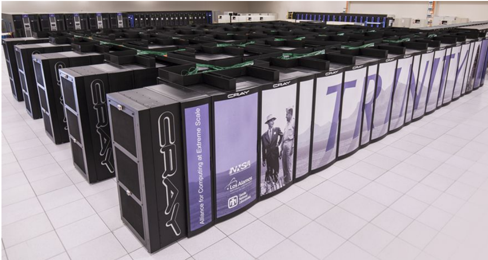
Trinity Supercomputer at Los Alamos National Laboratory
