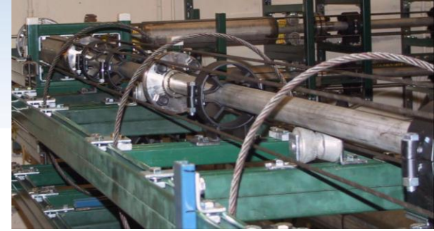
Piping and restraint cables
