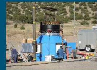
Custom 1000-gallon pressure vessel
