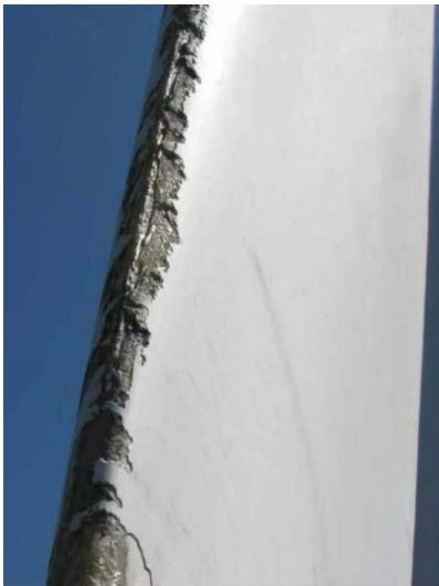
Heavy blade erosion 2
