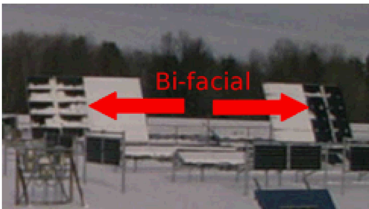
Figure 4. Time-stamped images of Trackers One and Two demonstrate that bifacial modules shed snow more quickly than the monofacial modules and that frameless modules (right) shed more quickly than framed (left).
