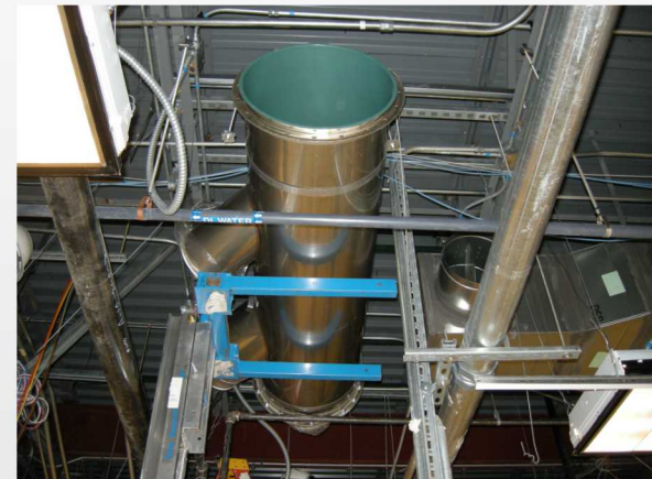
New PSP ductwork
