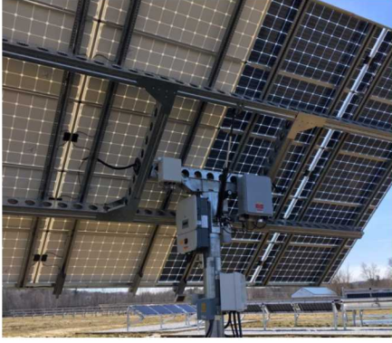
Figure 2. Backside of system one, with DC monitoring box and datalogger mounted on the pedestal. Monofacial modules are on the left side; bifacials on the right. Backside shading proved to have minimal impact on the bifacial gain for this system.
