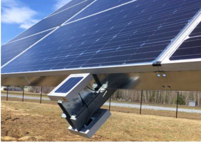
Figure 1 EETS reference cells mounted in the plane of array on both front and back of the tracker systems. The cells are cleaned twice a week.
