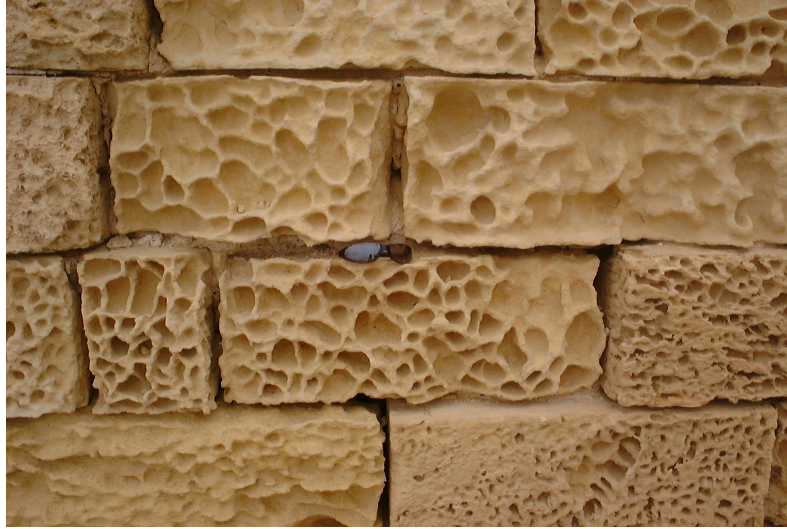
Fig. 6.1. Example of damage in building stones by crystallization of salts. (Photograph by Suzanne MacLeod, distributed under a CC-BY 2.0 license.)
