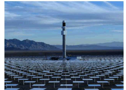
Crescent Dunes, molten salt, 110 MW e , NV, 2015
