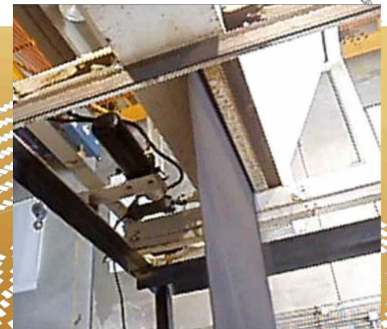
Falling Particle Receiver
