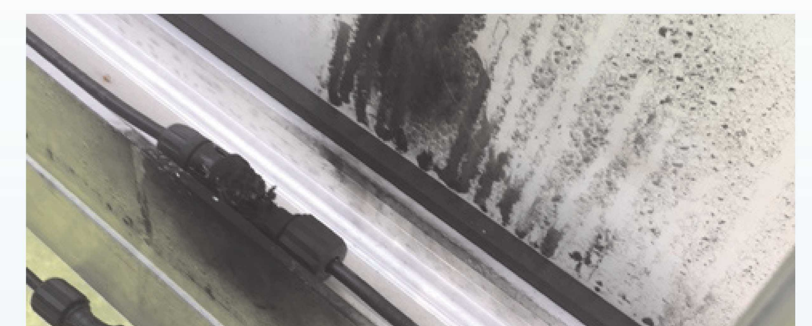
POOR INSTALLATION PRACTICES
