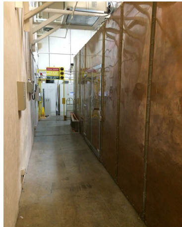
Photo 2: Standing inside double doors. Walking route that is leading to Test Cell & Shield Room
