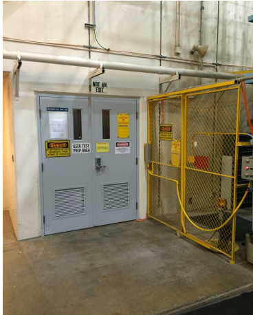
Photo 1: Entrance door into Controlled Area
