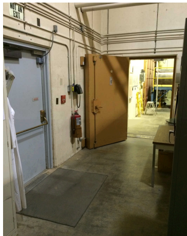
Photo 5: Shield Door (Door A) in open position.
