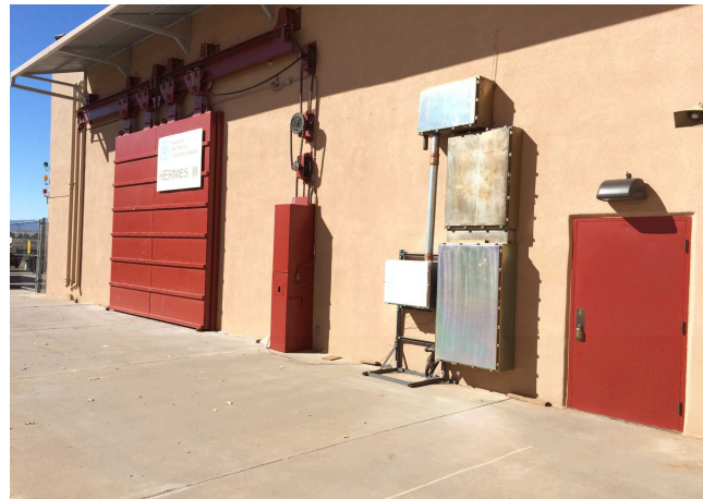
Photo 6: HERMES Courtyard. View of personnel entrance door (Door - B) and the test cell rolling door (Door - C).
