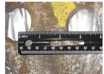
Carbon Steel Liner (Surrounding Heater)
