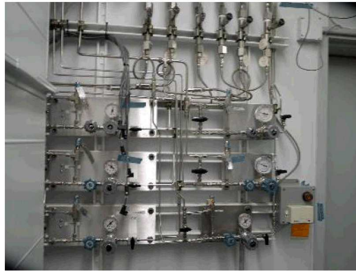
High pressure plumbing requires design and build and documentation of system for liquids and gasses
