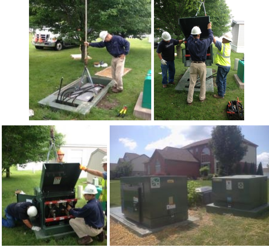
Figure 10: DTE CES system installation. In the bottom right photo, the CES is located to the left and the transformer is located on the right [9].
