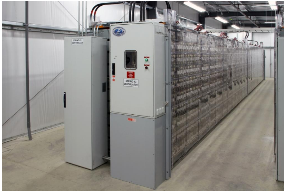
Figure 3: East Penn UltraBattery installation [3].
