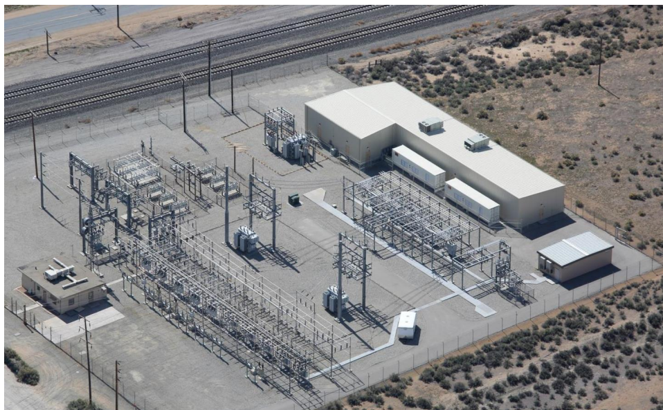
Figure 4: Tehachapi Wind Energy Storage plant, Tehachapi, CA [4].
