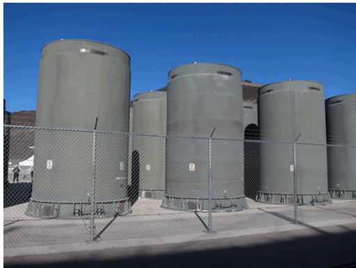
Diablo Canyon HI-STORM system
