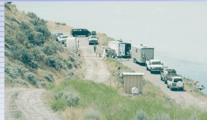
Injection of apatite forming solution at Hanford 100N site for immobilization of Sr-90. June, 2006.
