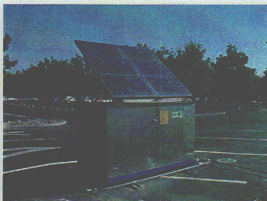
Solar-powered Treatment Unit (STU)
