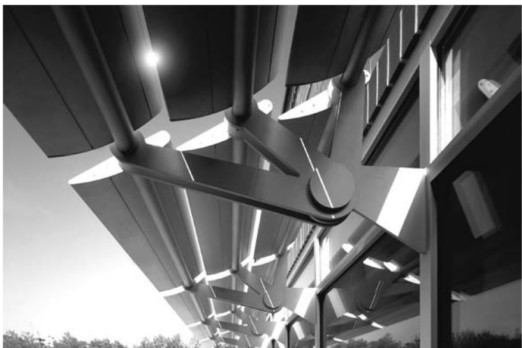
The PowerShade™ technology shades windows and generates electricity at EPA's lab complex in North Chelmsford, Massachusetts.
