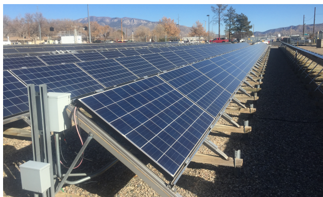
Fig. 1. The solar photovoltaic array was located in Albuquerque, New Mexico. It included two inverters that each supported four strings.
