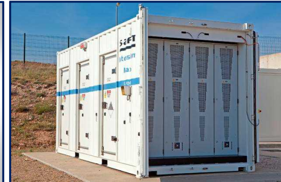
Utility Batteries (MWh)
