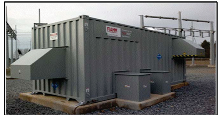
FIAMM 222-kWh System Duke Energy Rankin Substation
